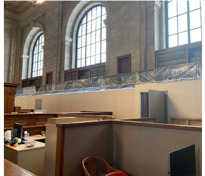
Bill Blass protection: Air handling units
